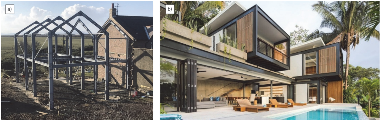
Figure 12. Examples of frame construction of family houses, a) Simple, repetitive frames [21], b) Costa Rica – urban steel villa [22]
