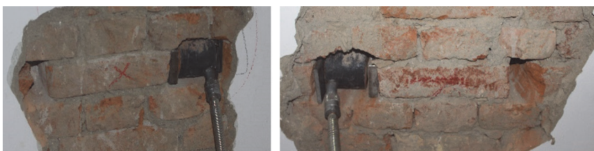
Figure 6. Residential building, Palmotičeva ulica 64a in Zagreb, masonry shear strength testing at locations PS-1-1 and PS-2-1
