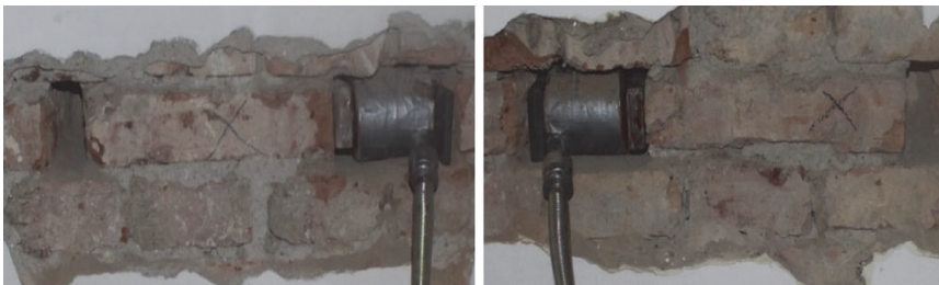
Figure 4. Office-residential building, Ulica Ivana Dežmana 9 in Zagreb, masonry shear strength testing at locations Z4 and Z6
