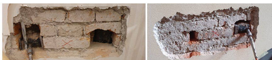
Figure 8. Hotel Palace, masonry shear strength testing at 1 st floor, at locations 1-1 and 1-7
