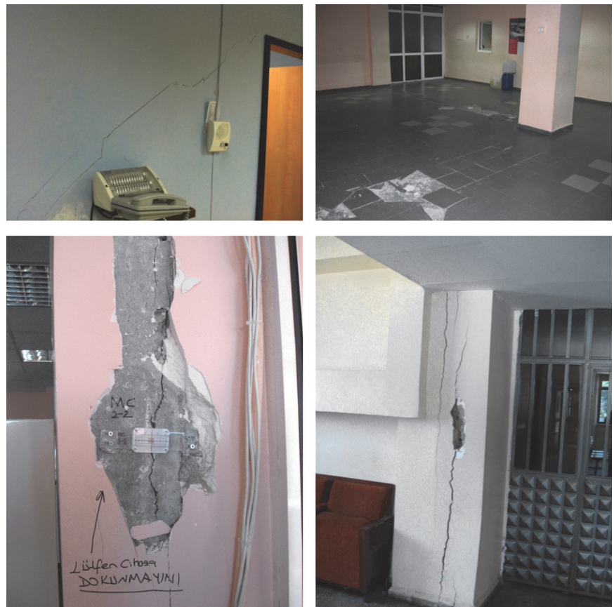
Figure 6. Cracking observed on structural and non-structural elements
